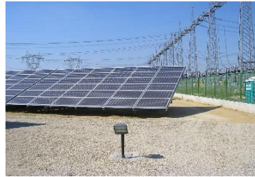
Several Region – 27 MW - TERNA
