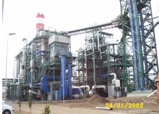
BIOMASS PP- 10 MW – CALABRIA Client: BIOMASSE ITALIA SPA
